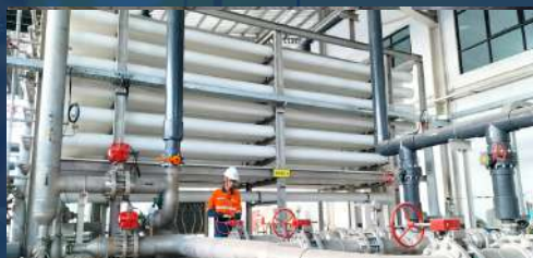
Desal-Demin Water Plant PT Amman Mineral Industri West Sumbawa Regency (operated by PT KTOP)
