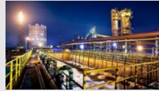
WWTP Biotreatment Blast Furnace PT KS 150 cmh
