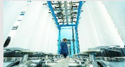
WRP & WTP Demin for PT LatinusaTbk 30 and 48 cmh
