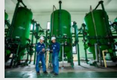
Demineralized Water Station Blast Furnace PT KS 150 cmh
