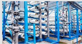
WTP Demin for PT MCCI 3 x 110 cmh
